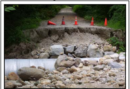
The floodwaters from the 2006 Mother's Day Storm tore a hole through Bartlett Loop road. Photo by Bridget Weber, FEMA.
