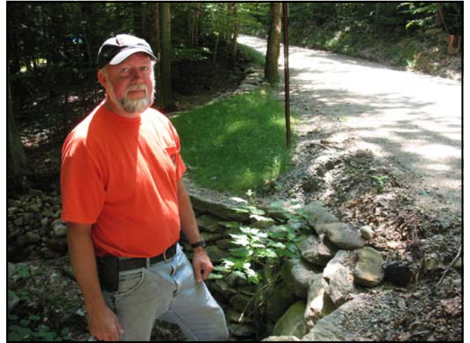
Road Agent Tim Fiske stands next to a repaired stone culvert on Fish Road where geotextiles were used in the roadbed. Photo Bridget Weber, FEMA.
