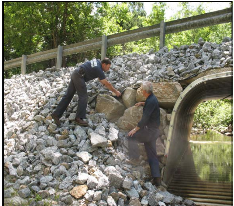
Emergency Management Director Edward Mical and Public Works Director Allan Brown show the placement of geosynthetic material in the roadbed of Bartlett Loop. Photo by Bridget Weber, FEMA.
